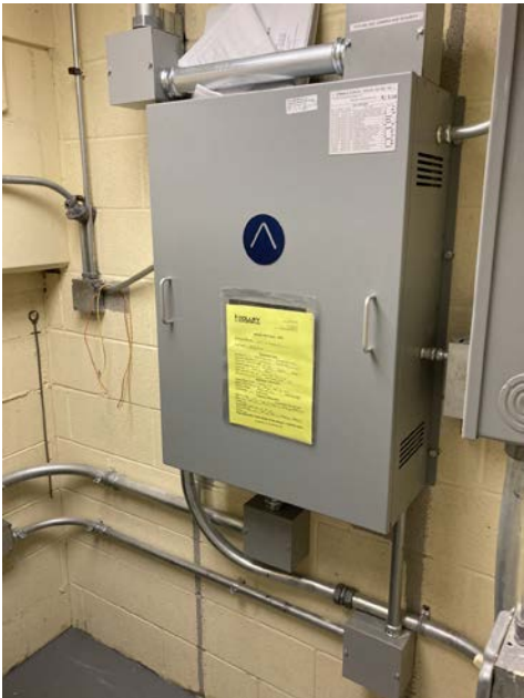
New elevator control board
