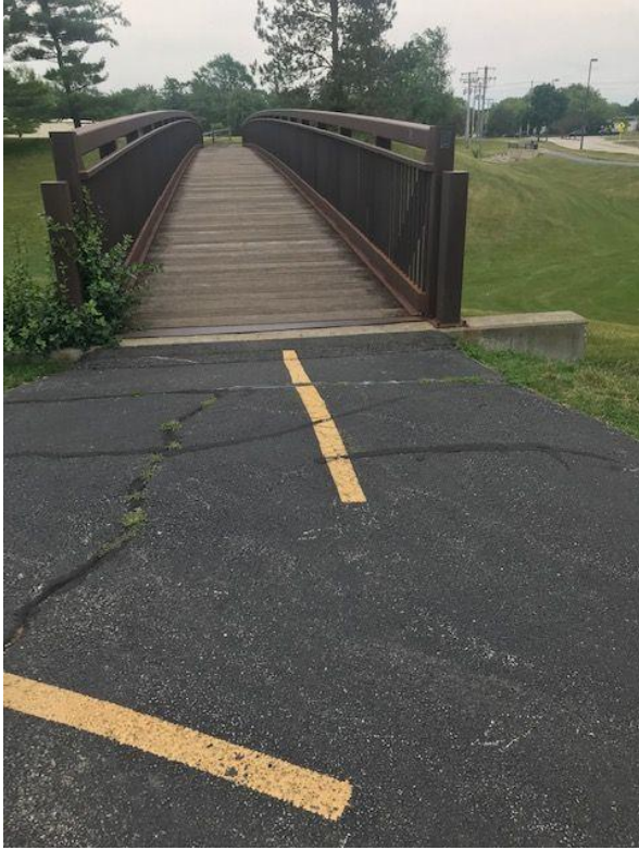
Bridge Approach before Repairs
